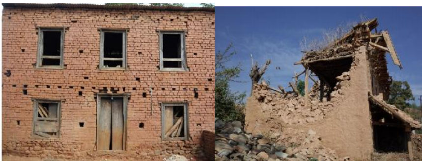
Figure 2. Difference of building damages between house materials Bricks and woods (left) and Muds and rocks (right)
