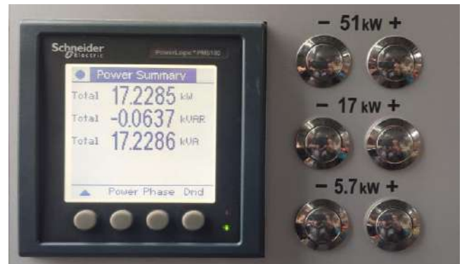
Figure 6. Control panel with power meter PM5110 series.
