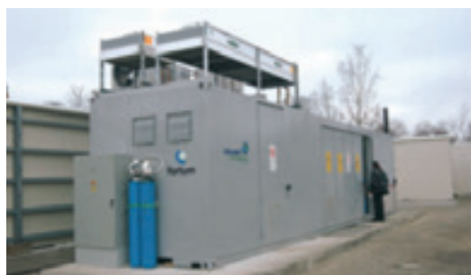
Figure 3. Hydrogen production plant (electrolyzer)
