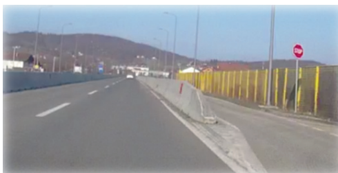
Figure 7. Unprotected new jersey barrier (M16.1)
