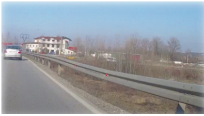
Figure 5. Poor maintenance (M16.1)
