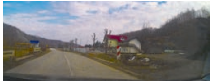
Figure 5. The lack of a protective fence on the bridge
