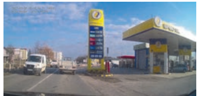
Figure 6. Unprotected steel structure of the gas station
