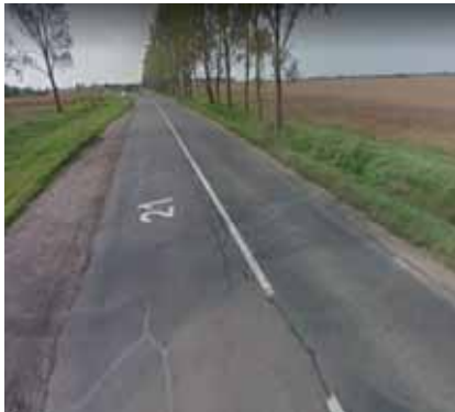
Figure 1. Separate segment of the existing variant of the section Ruma- Irig, where it is possible to change the horizontal signalization
