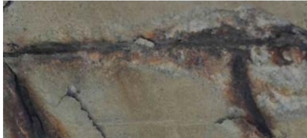
Picture 2. Degradation of concrete due to excessive chloride content
