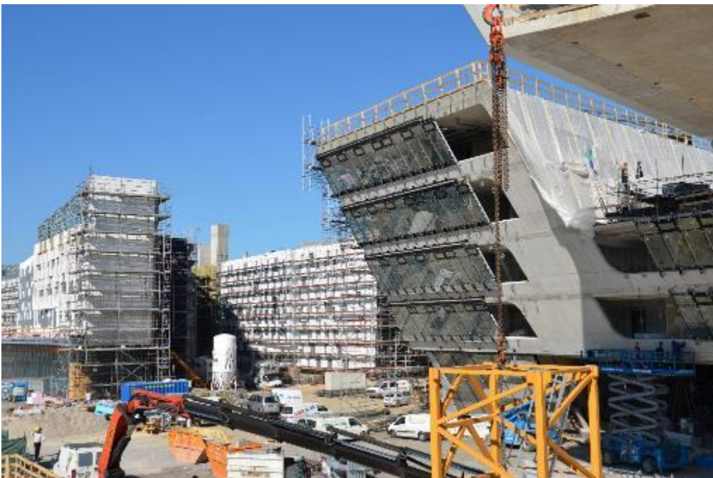
Fig. 1: Building site of the Campus of the Vienna University of Economics and Business, October 2012.
