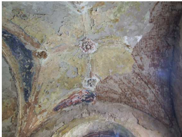
Figure 4. Damaged main entrance ceiling (Authors photograph from 2011.)
