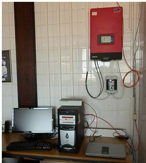
Figure 2. Part of the interior of the Solar energy laboratory at FSM in Niš with an inverter and additional equipment for monitoring and acquisition of data for 2 kW solar power plant
