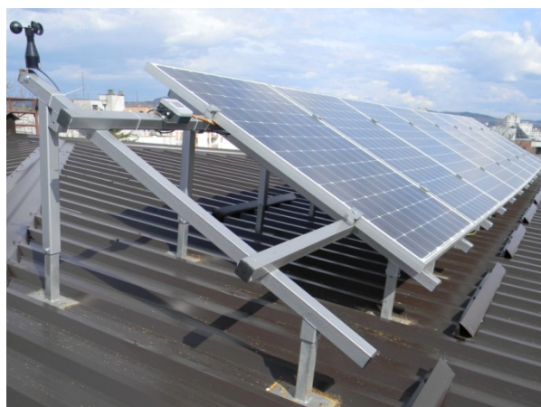
Figure 1. Solar system made of monocrystalline photovoltaic solar modules
