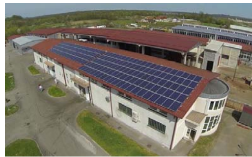
Figure 14. Rooftop on-grid PV solar plant of 50 kWp MI-TRAVIS
