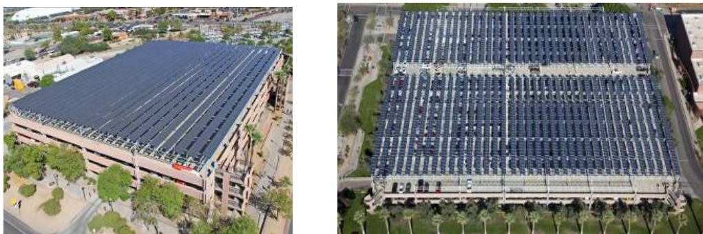
Figure 5. Arizona State University's photovoltaic installations are one of the largest commitments to solar energy by a University in the United States
