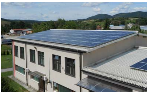
Figure 13. Rooftop on-grid PV solar plant of 50 kWp MADRA 2
