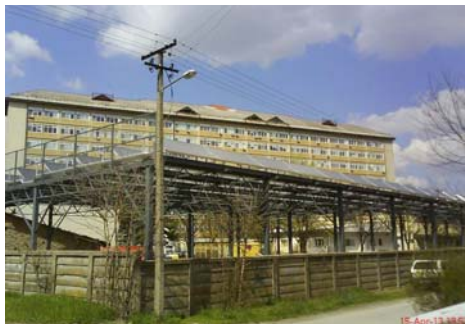
Figure 3. Hospital in Subotica, 144 collectors, 2013.
