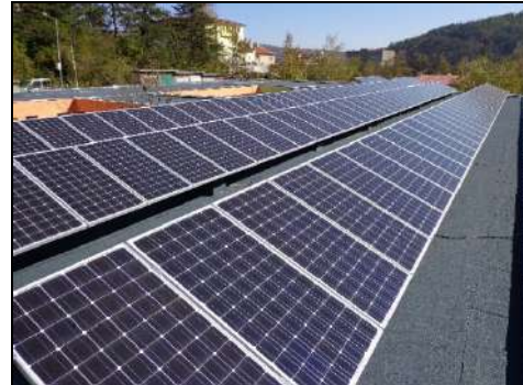
Figure 11. 23.76 kWp grid connected PV system on the roof of the kindergarten „First June“ in Gabrovo
