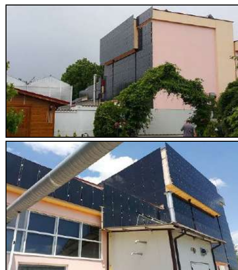
Figure 13. A 24 kWp CIGS photovoltaic facade power plant on the farm building [25]
