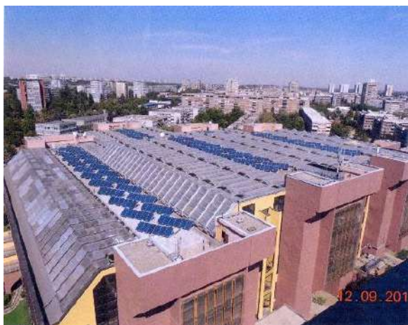
Figure 14. PV solar power plant on the roof of Energoprojekt in Belgrade, 115.62 kWp, 2013.
