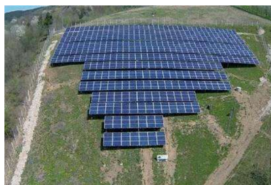
Figure 17. 249 kWp PV solar power plant Novaković-besjeda in Vijačani village, Prnjavor, 2014.
