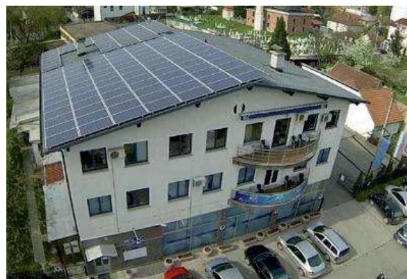
Figure 16. 20 kWp PV solar power plant BLC 1 (2012) and 10 kWp PV solar power plant BLC 2, (2014) Banja Luka
