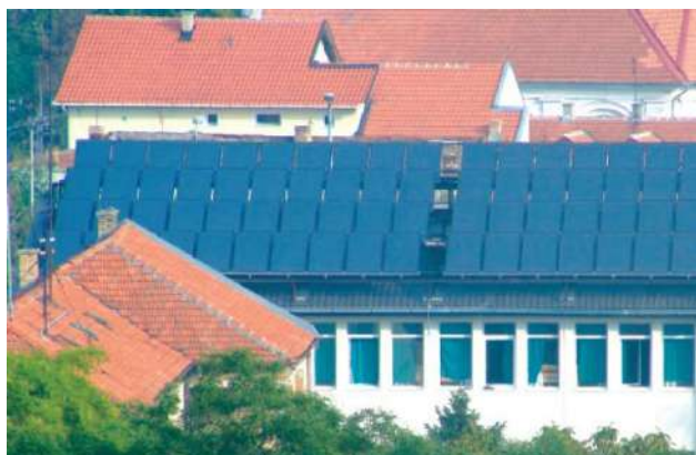
Figure 10. Solar collectors on the roof of the Residence Hall „Angelina Kojić-Gina” in Zrenjanin
